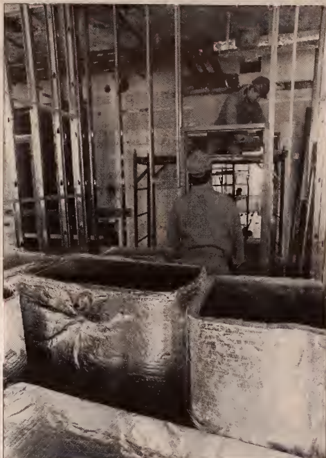
From the inside out . . . Two workers from the Office of Physical Plant's renovation crew work inside the gutted Weaver Building at University Park. The $2.1 million facelift, funded by the University's Capital Improvement Fund and state money provided by Operation Jump Start, includes work to both the interior and the exterior of the 80-year-old structure. For more photos and information, see page 15. Photo: Greg Grieco
